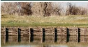
Water channelization & degradation
